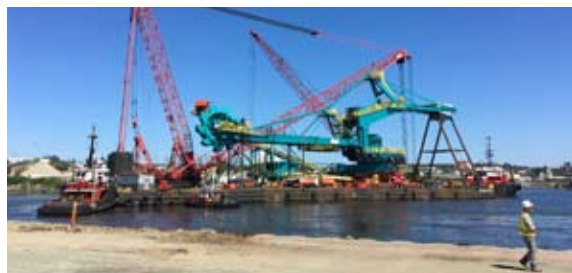
Fully assembled Stacker-Reclaimer being delivered on 'Dynamic Beast' from Victoria to Vancouver
